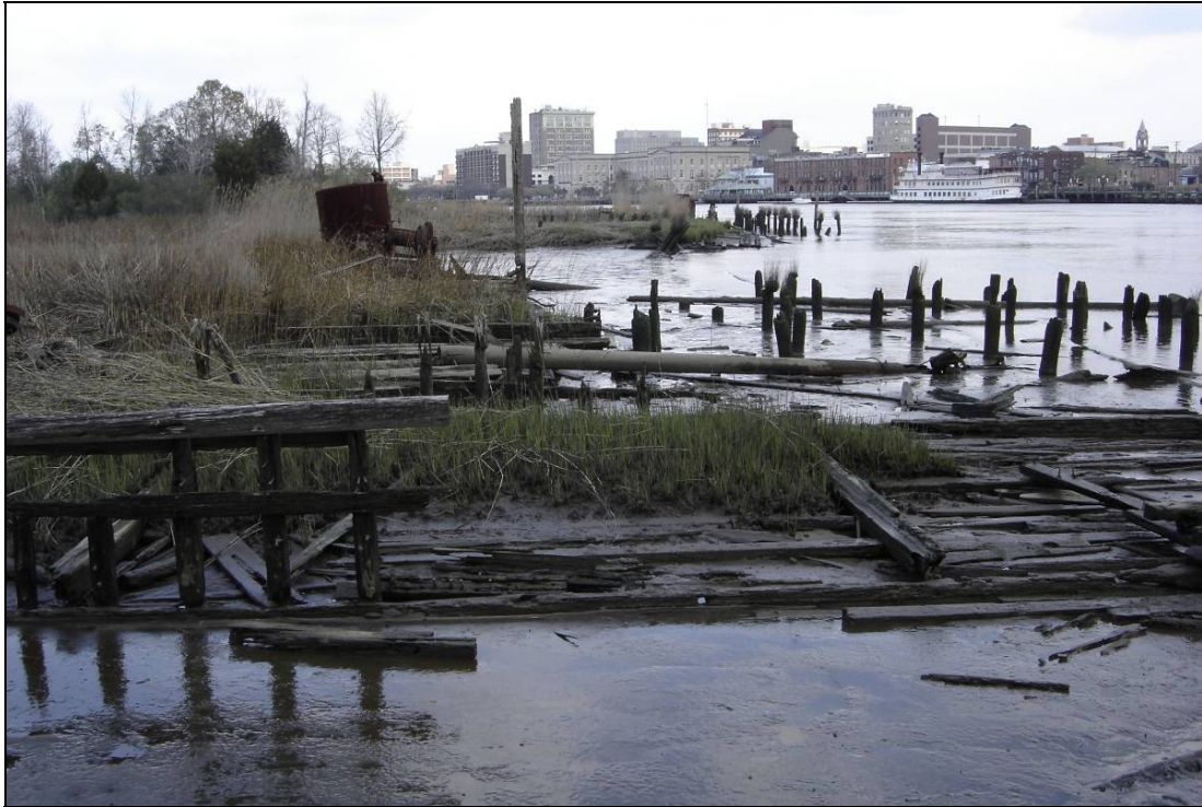
Figure 7.6: The cluster of four barges is lined, on the river side (east) with piles indicating likely reuse in association with a dock structure (Image by Amy Leuchtmann).
