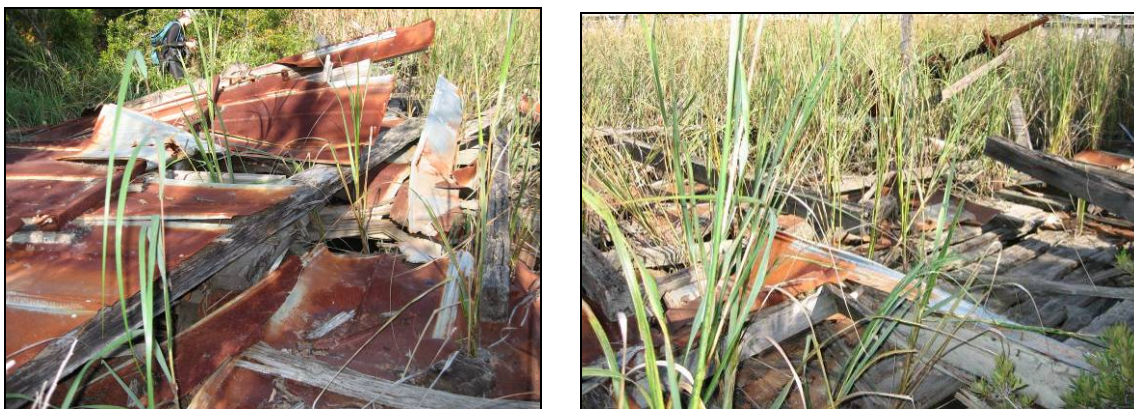
Figure 6.11: Collapsed Carpentry Shop in the Stone Towing and Marine Railway yard, north of Stockpile 2 (Images by author).
