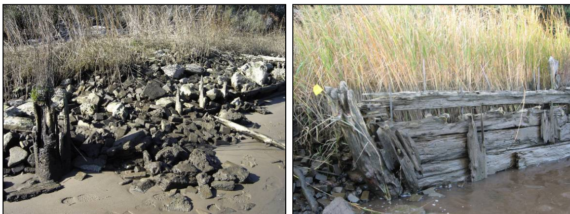
Figure 8.12: Examples of placement assurance. (Left) Bulkhead tug filled with rock and brick debris and (right) Bulkhead Barge, likely filled with dredge spoil (Images by author).
