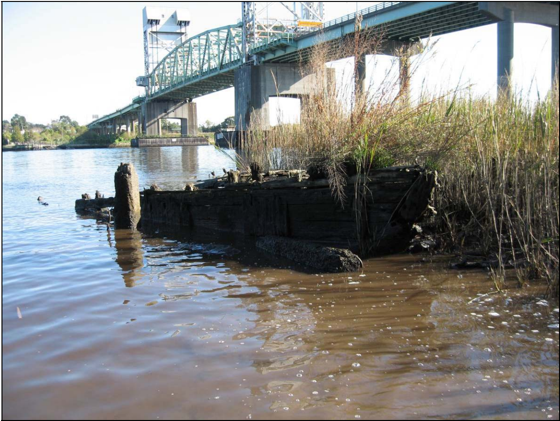
Figure 8.15: Concrete piles (one has fallen) on the north side of the Government Barge might be a signature of placement assurance (Image by author).
